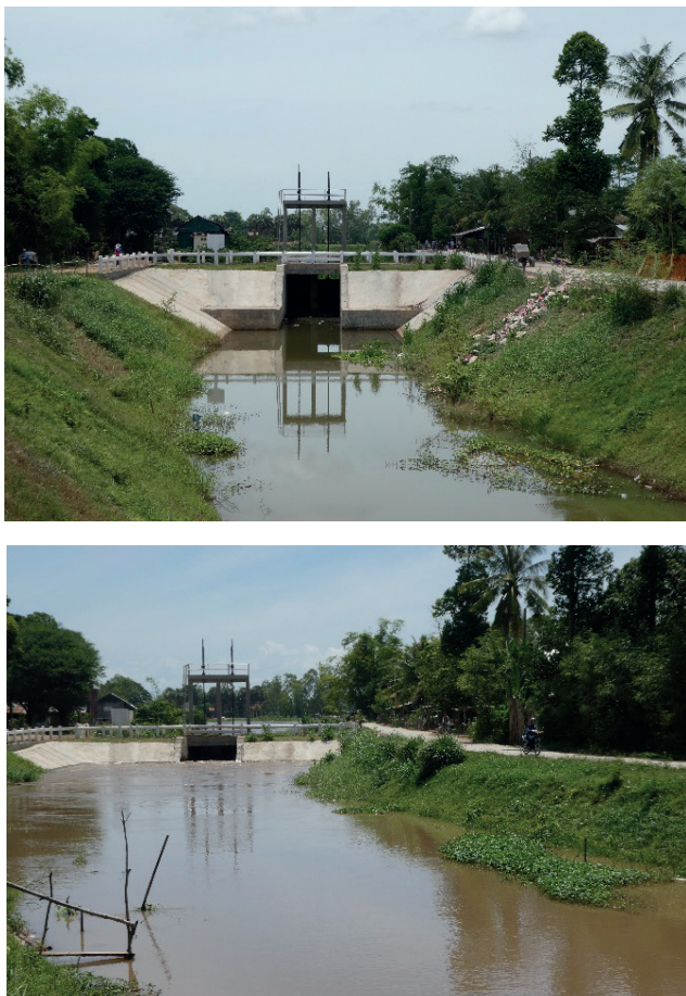
Figure 4. Example of sluice gates built under the AFD funded WASP project (Left: June 2017; right: September 2017; Credit: Jean-Philippe Venot)
