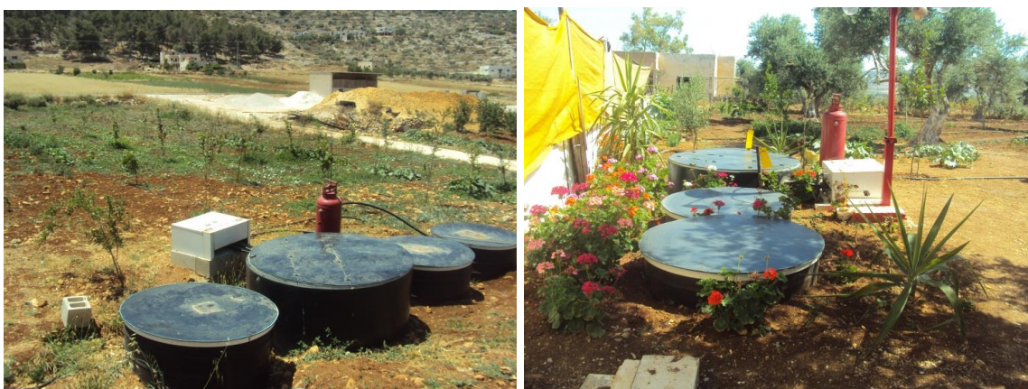
PHOTO 2.4: ARIJ'S SMALL SCALE ONSITE WASTEWATER TREATMENT PLANTS
