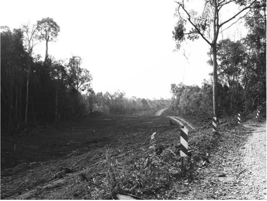
Figure 4.5 Excessive road clearance
